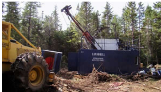
Drilling activities on Hole 10 - 4 on the West Zone of the Mooseland Gold Project.
