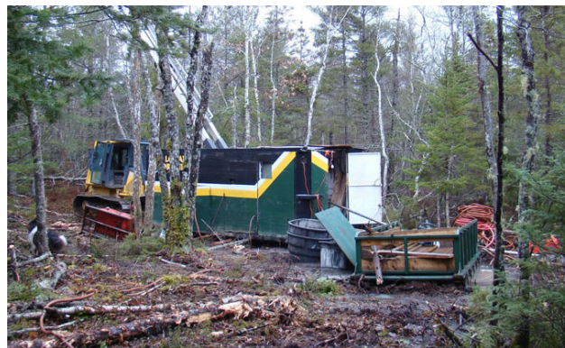
Late 2010, three diamond drill holes were completed at Leipsigate which gave NSGold's geologists a better understanding of the area and a target for further exploration.
