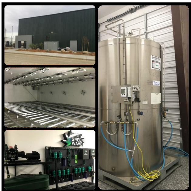
Next Green wave has already completed the installation of dehumidifiers, lights, rolling benches, irrigation manifolds, water filtration, security and Co2 distribution systems.
