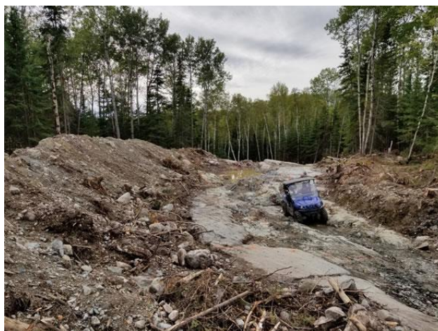
Part of the Francoeur property that was stripped from overburden and pressure washed to expose the bedrock.
