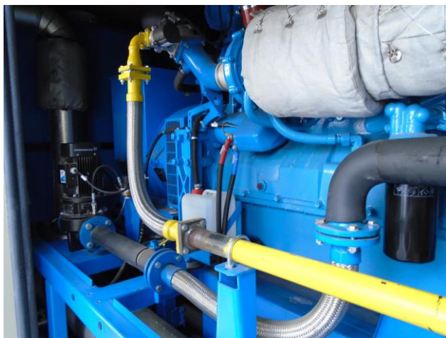
Part of a CHP unit's natural gas engine.
