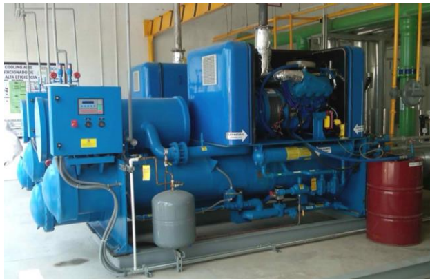
A gas-engine driven chiller in operation. The proven engine design of these chillers, have over 80 million hours of reliable operation.
