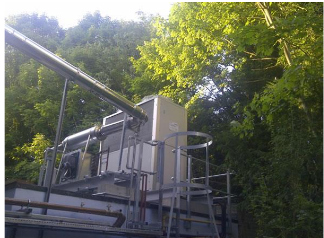
Part of the gas heat pump at the Haverhill Leisure Centre in Suffolk, UK.
