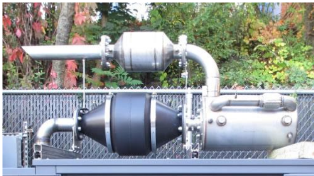
The Ultra Emissions System mounted on top of a CHP unit.
