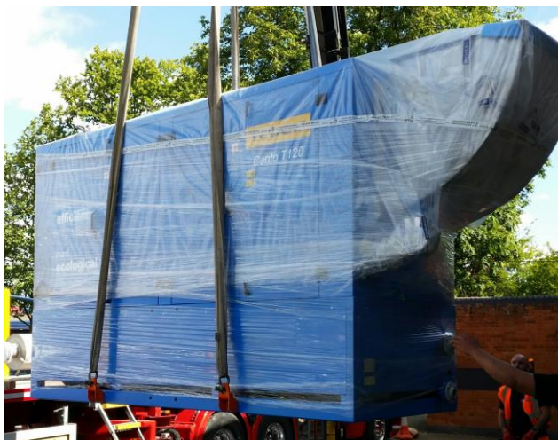
The Combined Heat & Power system being delivered at the Kingfisher Leisure Centre.
