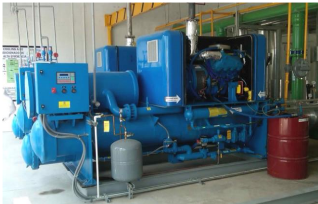
A gas-engine driven chiller in operation. The proven engine design of these chillers, have over 80 million hours of reliable operation.
