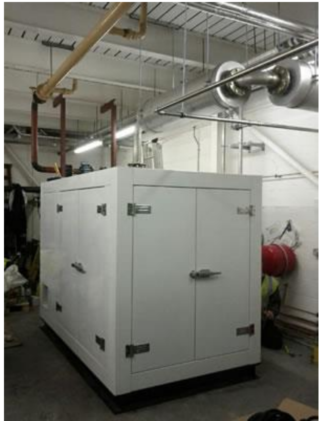
Combined Heat and Power systems, such as this one at the Roko Health Club in Portsmouth, use fuel very efficiently, as they provide electricity and heat at a combined efficiency approaching 90%.
