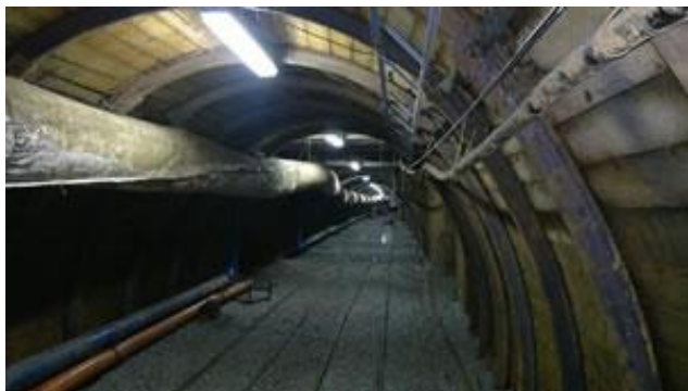
Part of the dewatered and rehabilitated tunnel at Level 6 (approximately 180 metres below surface).
