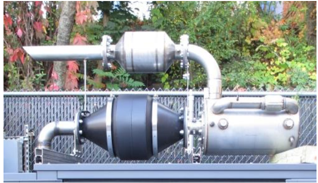
The Ultera Emissions System mounted to a CHP unit. The Ultera is designed to deliver simple, cost-effective solutions for natural gas engines to meet stringent emissions standards.
